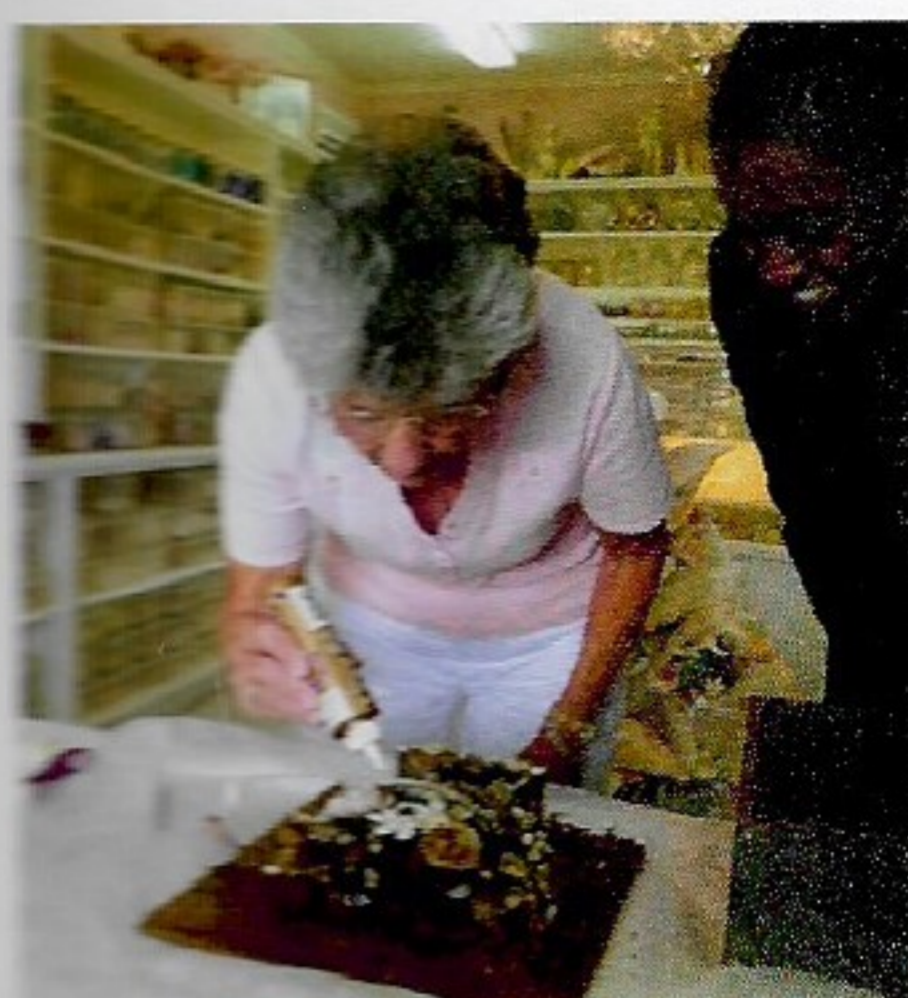
Daphne Hunte repairing the shell work at the Curator Art/Art History Allison Callender looks on
